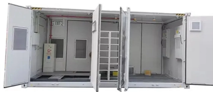
1075KW HH ESS
